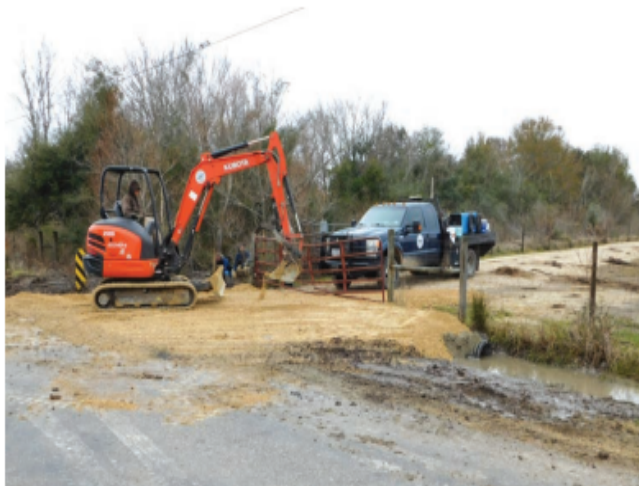
DD6 workers finish up a private road built in exchange for easement.
