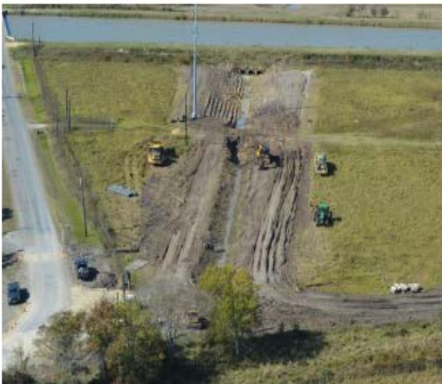
DD6 workers prepare to widen this ditch crossing from one smaller pipe to three larger pipes.
